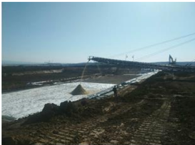
Fig.4: Gypsum dump location in the excavated area of the open cast mine Drmno
