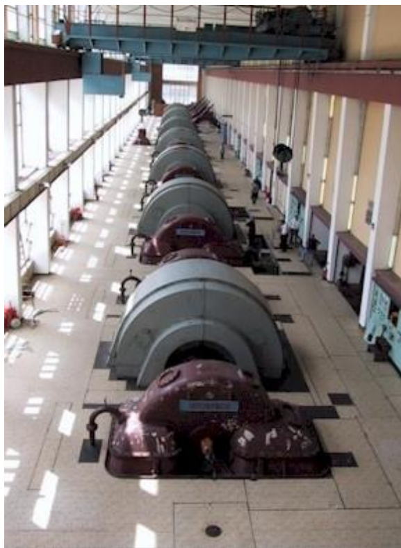
Fig. 7: Perućica HPP powerhouse with seven Pelton turbine units
