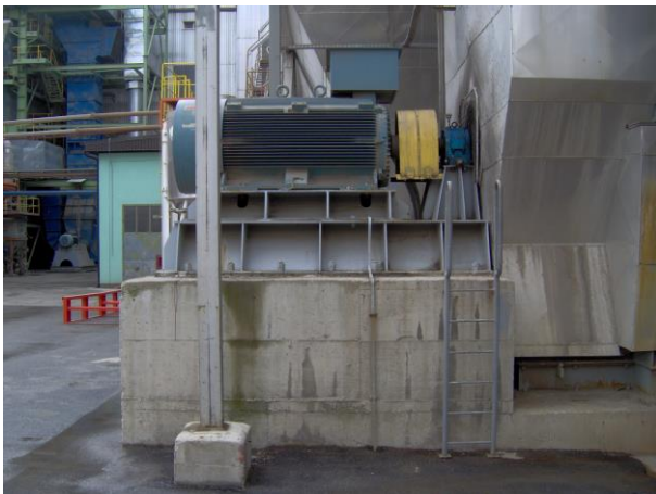
Fig.1: Motor flexibly coupled with ventilator
