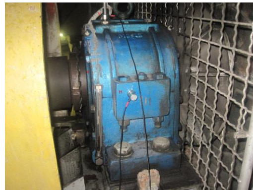
Fig.5: Bearing housing with accelerometer attached
