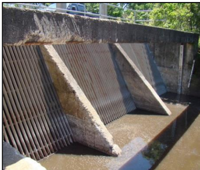
Fig.1: Trash rack at the intake of the hydropower plant (wilcoxdiving.com).
